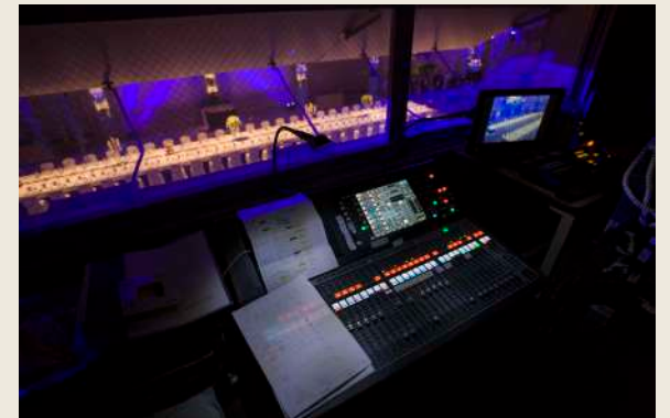
Audio Equipment | 音響設備
